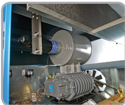
View with rear panels removed
